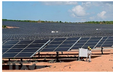
Solar power plant becomes operational in Ninh Thuan
